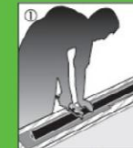
All pipe penetrations, first cut a piece of BIKUPLAN® KSK triangular fillet to the required length.
